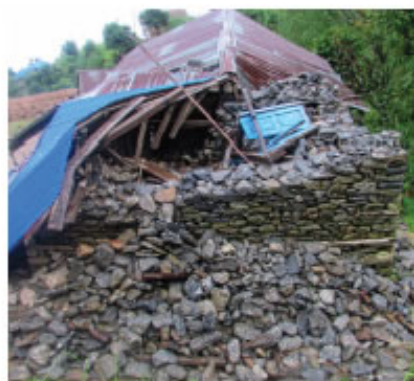
Yuba Jyoti Primary School, Dipsung. D2N purchased the land the school was constructed on. This is one of the schools being rebuilt.
